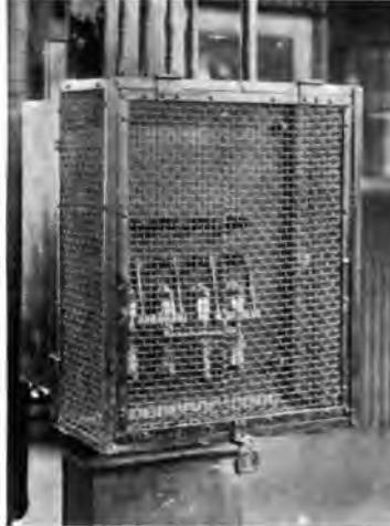
Fig. 2. Switch Enclosure in Plant.
